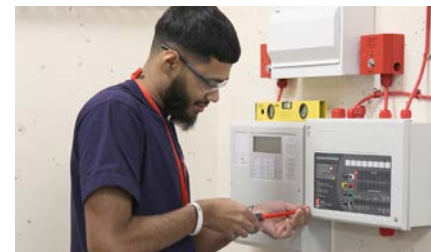
Fire and Security
